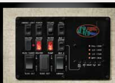
SIERRA's control center allows you to monitor tanks and other systems quickly and easily.
